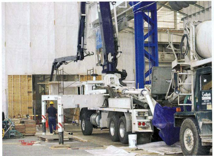
For the safety of manufacturing facility workers present throughout the Boeing floor demo and replacement project, Healy, Long & Jevin outfitted its equipment with exhaust scrubbers, including a bolt-on model for its concrete pump truck.
